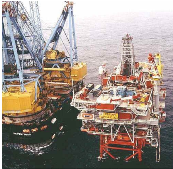
A giant floating crane used to build the Captain Oil production platform it dwarfs the actual platform
